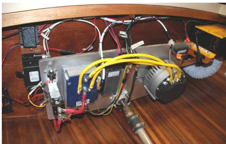
The launch's tidy motor and PMAC unit
